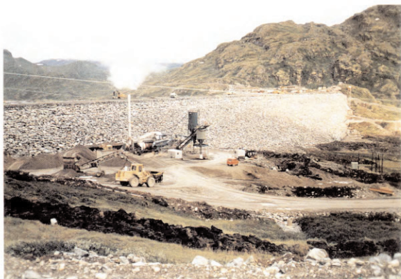
Fig. 4.2 The batch plant erected close to the downstream toe of Riskallvatn Dam
