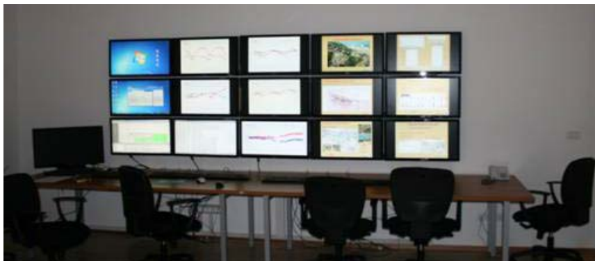
Figure 38: Monitoring room at the Ancona landslide EW Centre.
