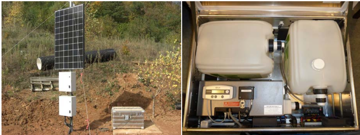
Figure 31: Left: Monitoring system with fuel cell and solar panel. Right: Fuel cell with 2x28 l methanol canisters and GSM modem.
